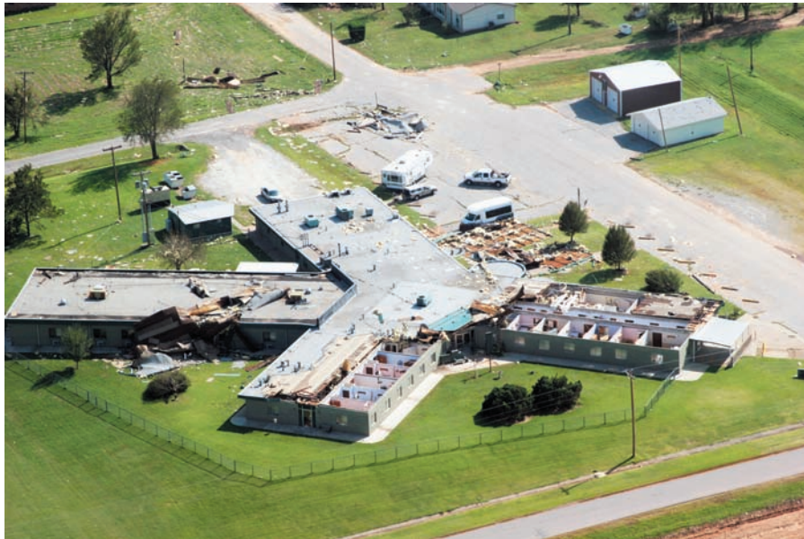
Plate 8.2. Caddo County, Oklahoma, August 20, 2007 – Damage to a nursing home as a result of a tropical storm. There were no injuries. Patricia Brach/FEMA News Photo.
